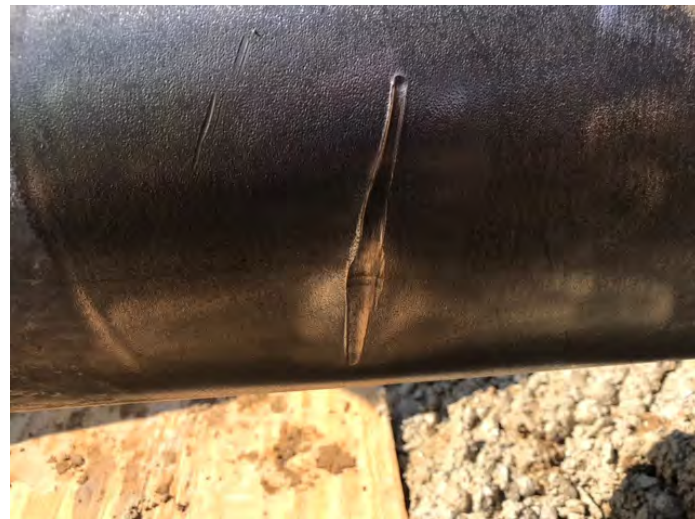
This scratch was discovered during an excavation on an existing 12" natural gas line. The pipeline was excavated where the scratch was discovered and reported to the owning client. It is unknown when the scratch occurred or how. It is suspected that the damage came from a tiger tooth on a bucket or an improperly installed flat bar welded on teeth. Area work was halted and repairs were scheduled immediately. Unknown metal loss amount. Unknown remaining wall thickness.
