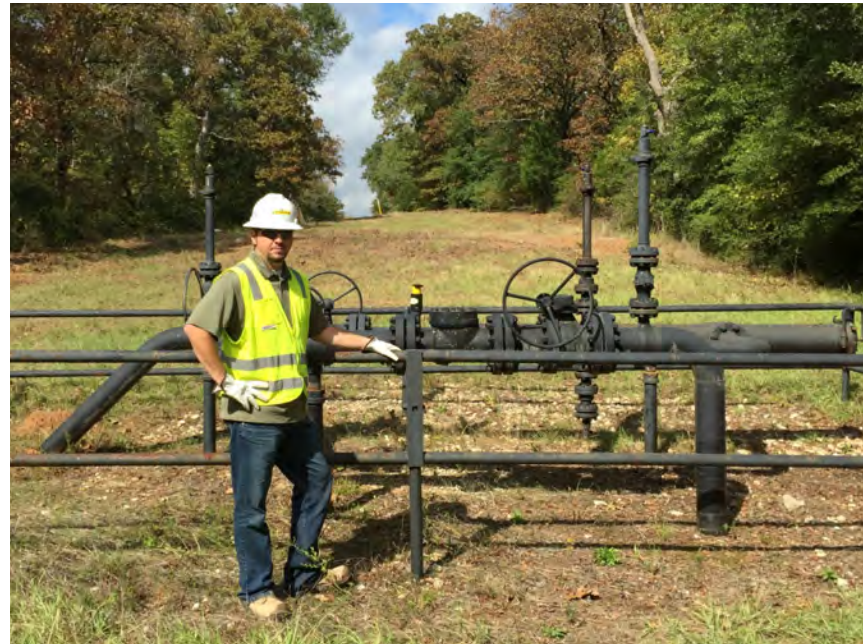
Here was a pipeline patrol Patriot Pipeline conducted on a gathering system in east Texas. They developed a comprehensive report to identify security vulnerabilities, corrosion detail, quality assessments, and CFR compliance assessments.
